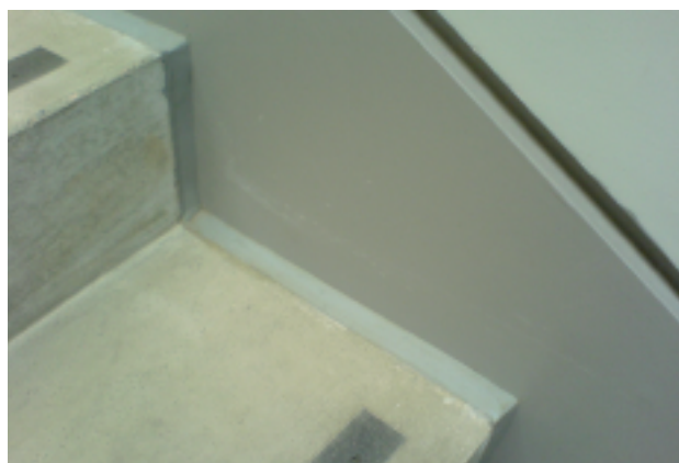
▲ Above a mastic joint and mdf skirting fills the construction joint between a self-finish pre-cast concrete stair and the wall
