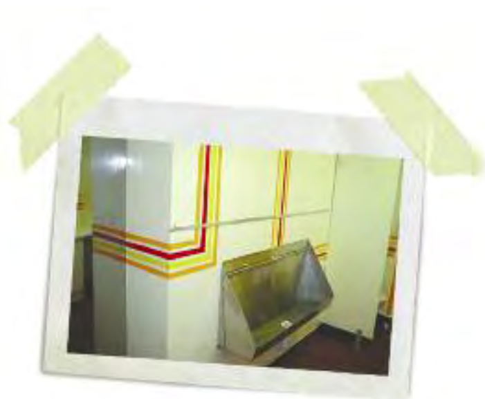
▲ Above trough urinals should be avoided
